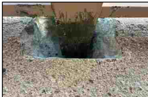
CHIPPING OF RAILING POST POCKETS
