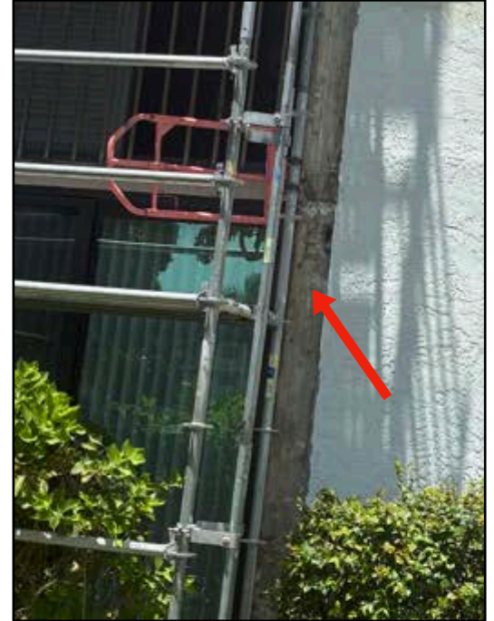
Column Repair needed / building 30 Exposed rebar.
