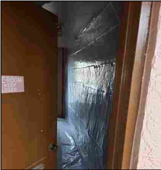
Dust walls installed in storage rooms
