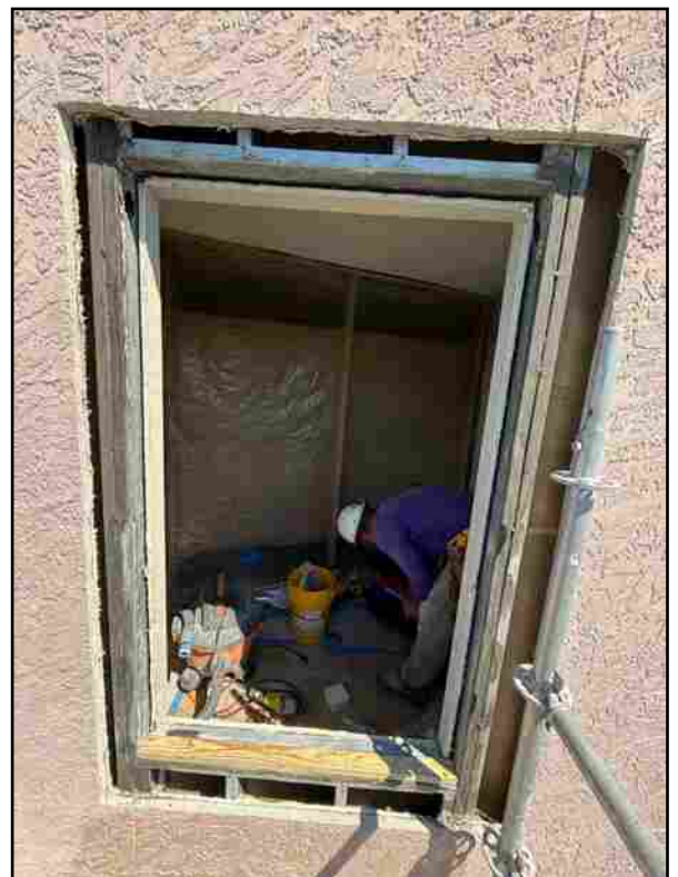
Rusted window frame
