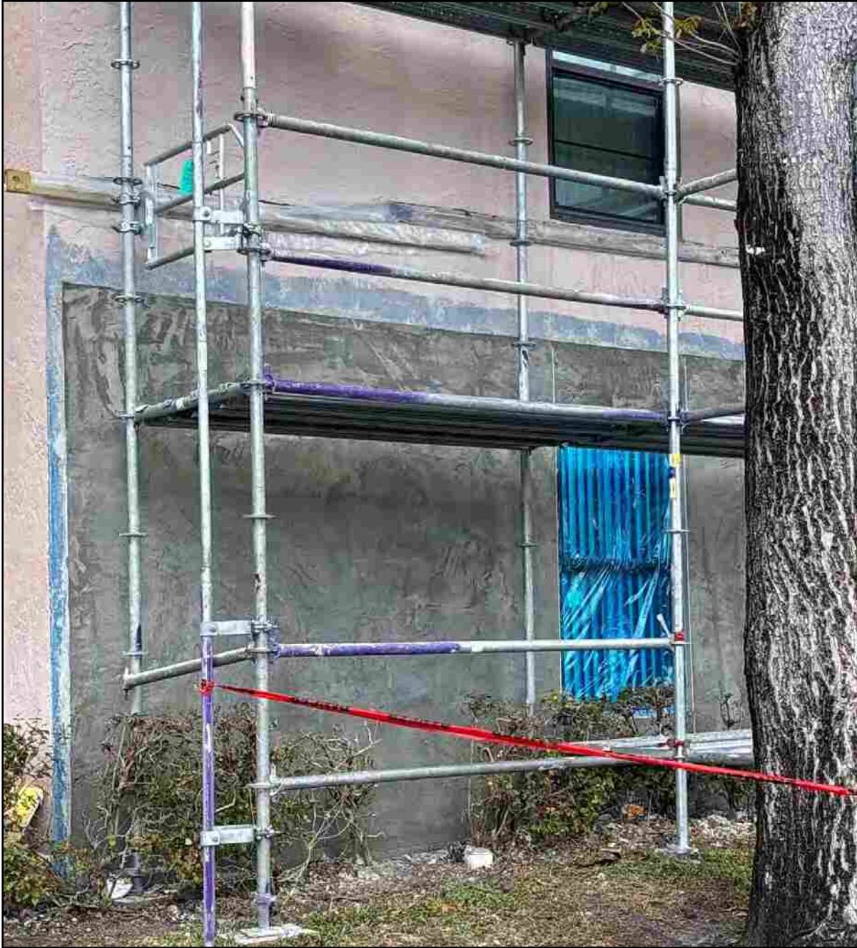
Stucco on EFIS system BLDG 31 Unit 110
